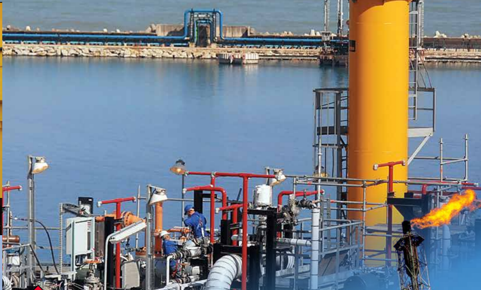
7.6t x 15m Box Jib Cranes - Entrepouse Contracting New LNG Train Skikda, Algeria
